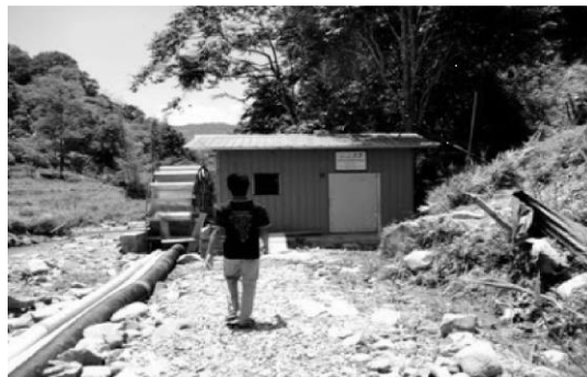
Figure 3: Mini Hydro Electric Generator by Mr. Abdul Hamid Jasmin
